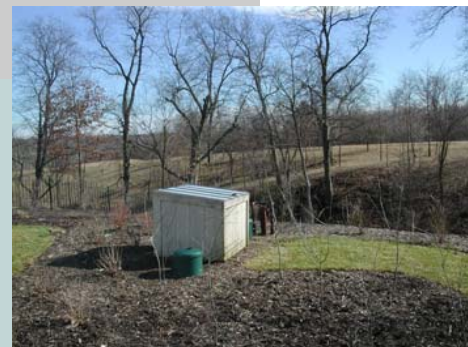
An experimental Drip Home Sewage Treatment System
